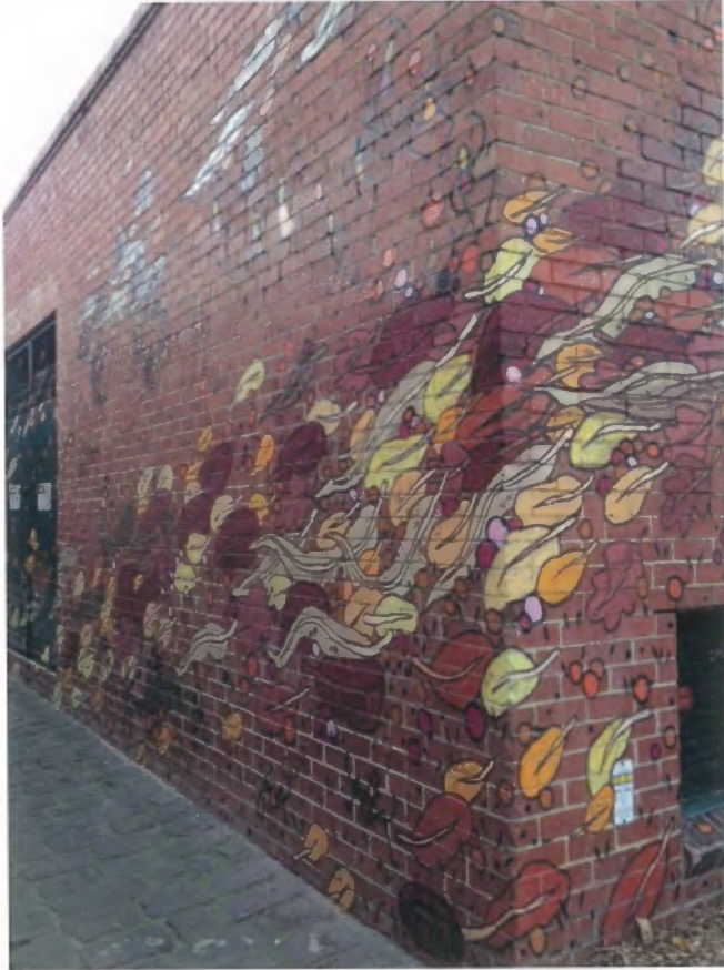
The colourful mural on the wall of the electricity substation. The mural makes the whole space brighter and discourages tagging and graffiti.
